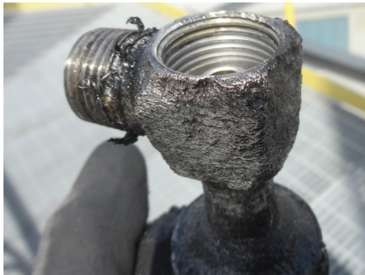
Figure 6. Fouled spray lance.
