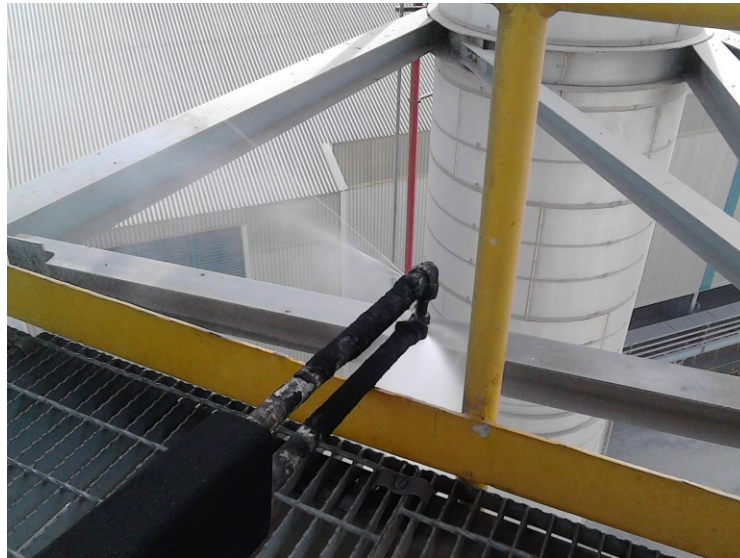
Figure 5. Inspection of lance spray with faulty pattern.
