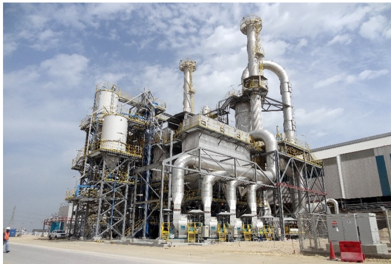
Figure 1. Pleno V Fume Treatment Center.
